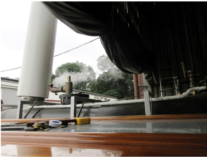
Safety valve starting to lift
