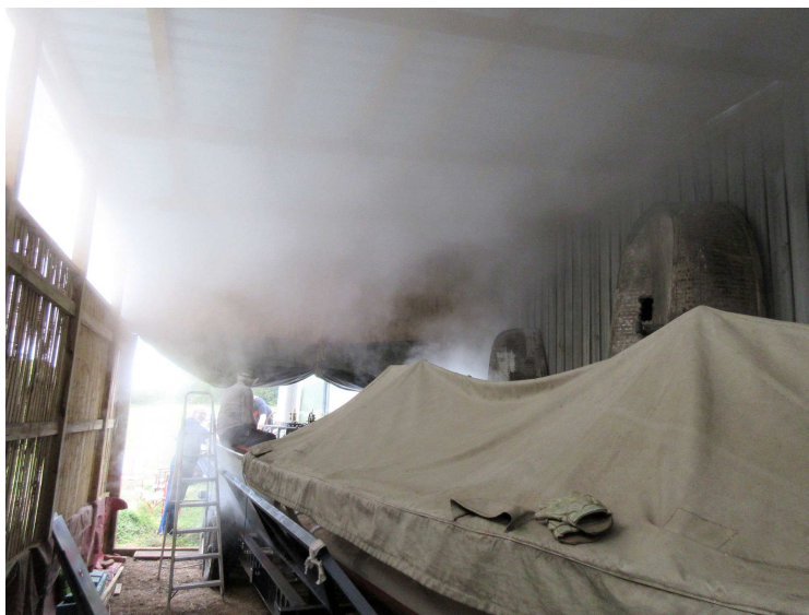
A lot of steam was blown into the shed during the boiler blow down even though the skin fitting was outside.
